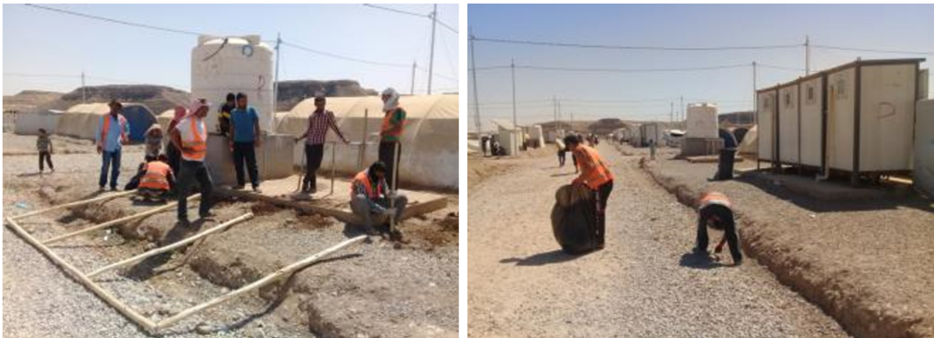
Left: Workers engaged in the installation of privacy screens in Hasansham M2 IDPs camp, Ninewah. Right: Workers cleaning a drainage channel in Hasansham M2 IDPs camp, Ninewah
